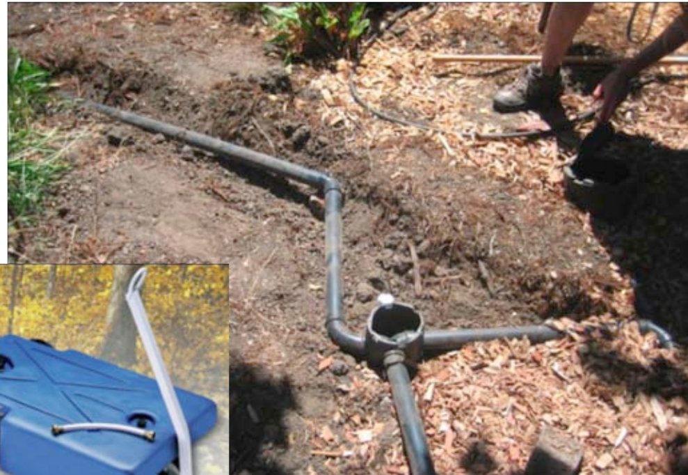
Branched drain system
