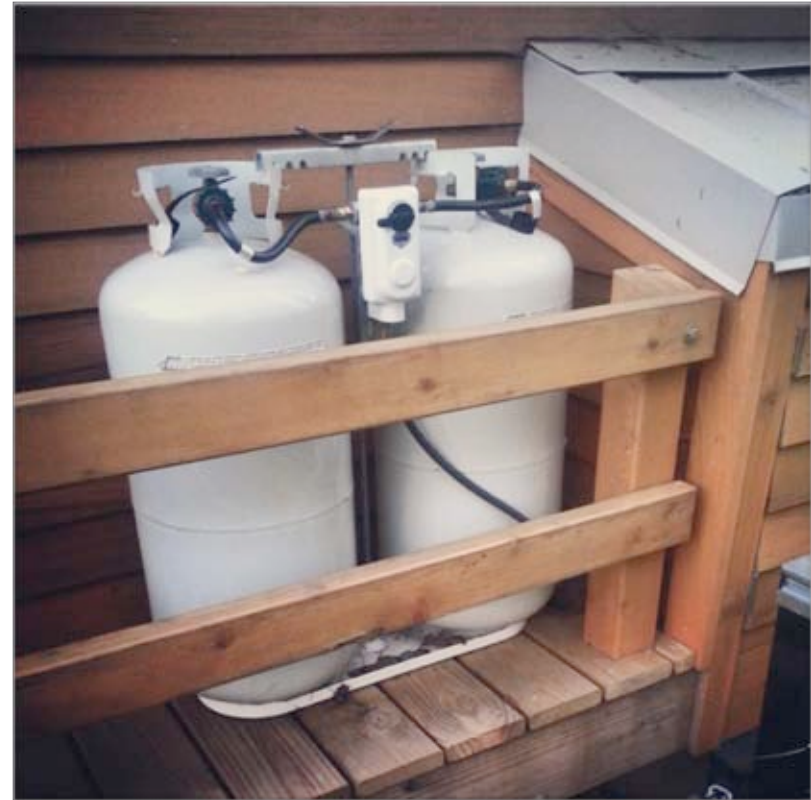
Our 2 40 gallon propane tanks and regulator
