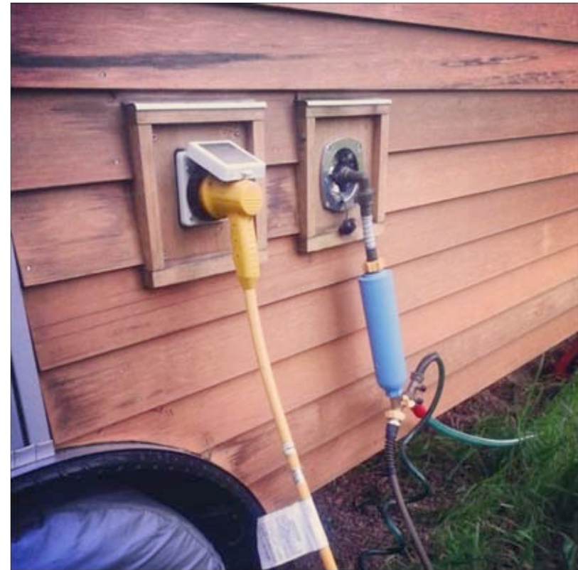
The Tiny Project 30-amp RV power hookup
