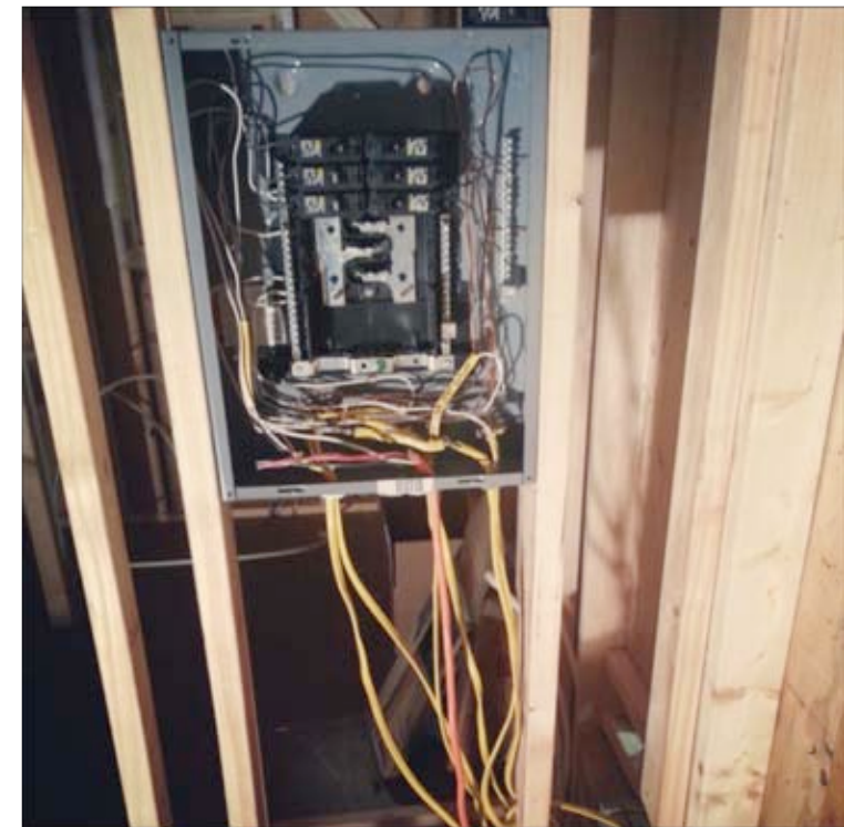
Our electrical panel
